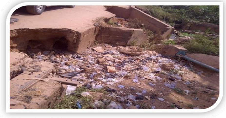
Plate 2: Improper disposal of waste into the drainage channel causing flood in Banawa Area. Source: Authors fieldwork, 2022.
