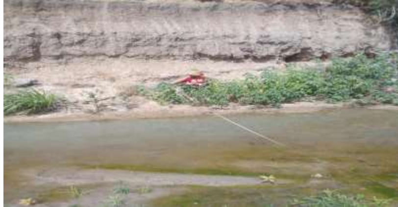
Plate 1: Collapse of Dongol stream side walls due to mass wasting process
